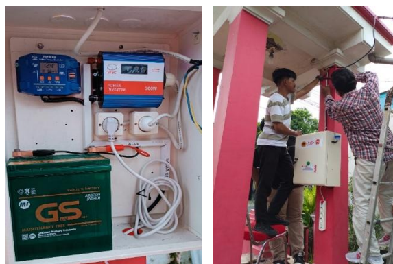
Figure 5. Implementation of Street Lights and Panels for Lighting Around Gaprang Village Hall
