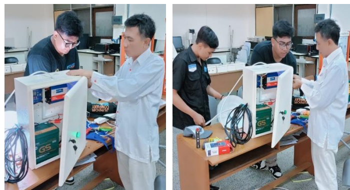
Figure 4. Solar Charge Control (SCC), Battery, and Inverter Installation
